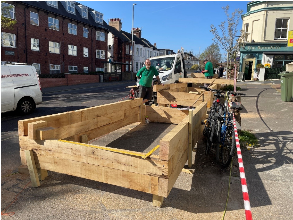
April 2025: Construction of the Prince's Crescent biodiversity planters. The scheme was delivered through collaboration between local volunteers, contractors and project partners, transforming underused streetscape into community-managed green infrastructure.
